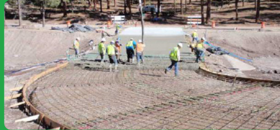
Location: Santa Clara, NM Client: Federal Highway Administration Project: Concrete Rigid Paving
